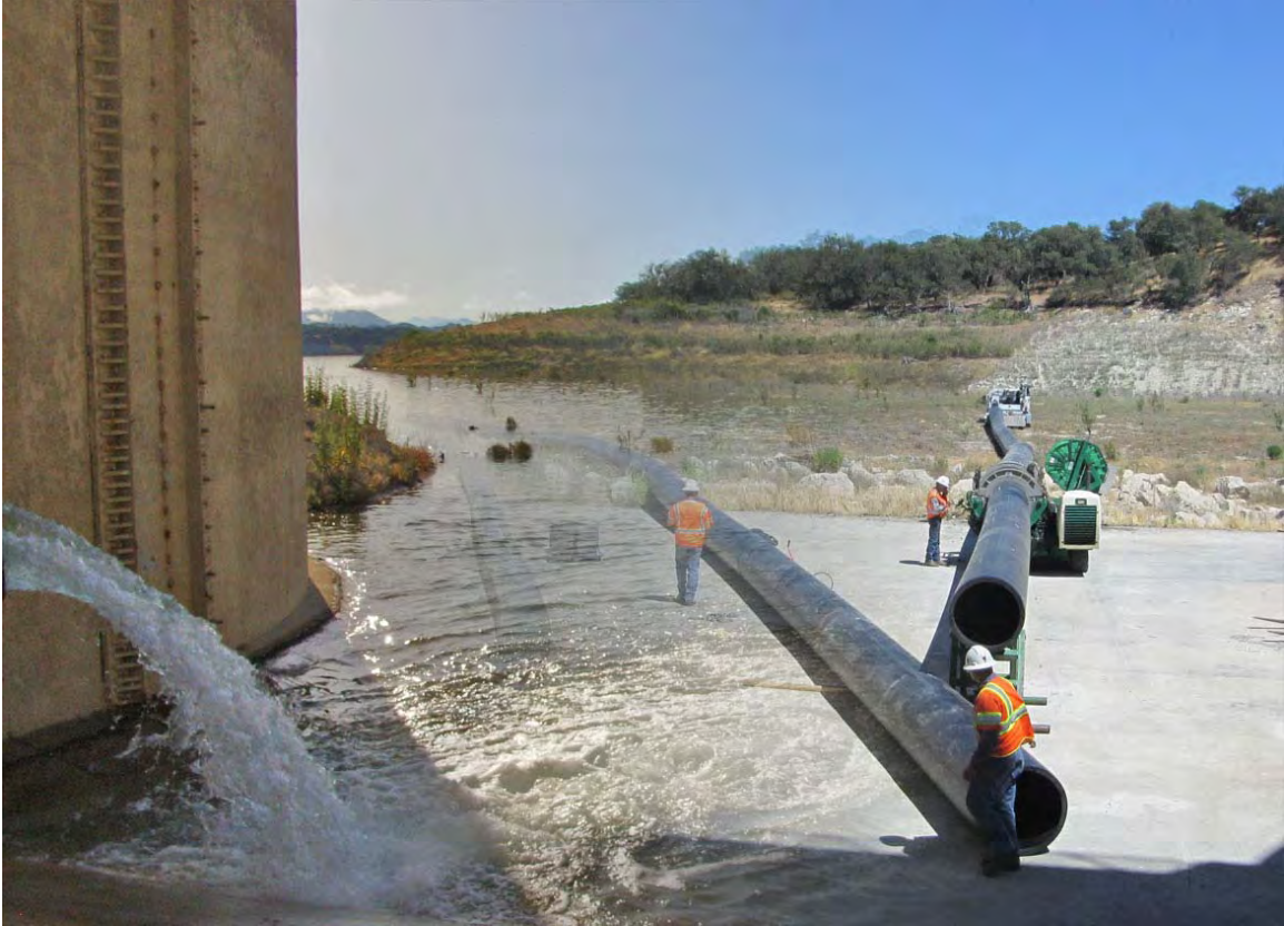
Bypass Piping at Bradbury Dam 2017 vs 2016
