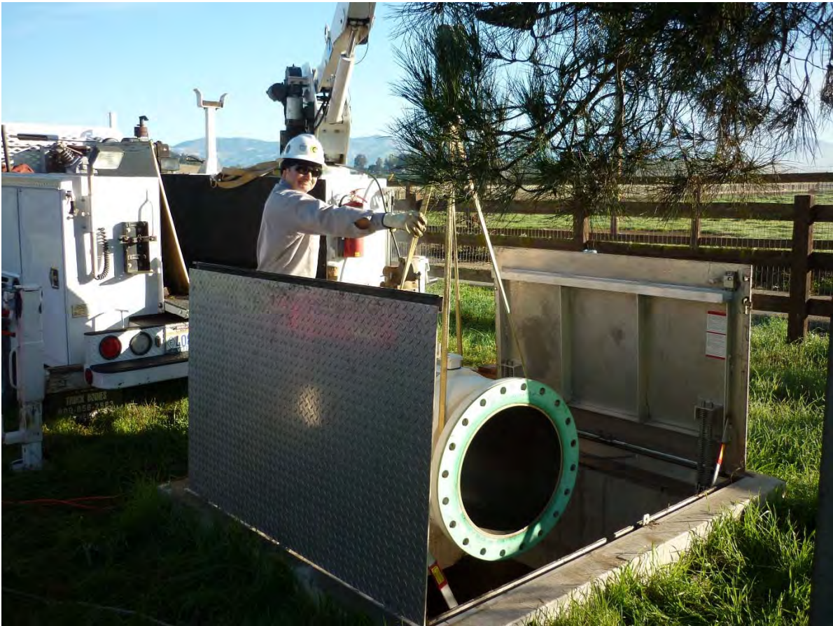
Removing ABB Flow Element during February 2017 Shutdown of Santa Ynez Pumping Plant
